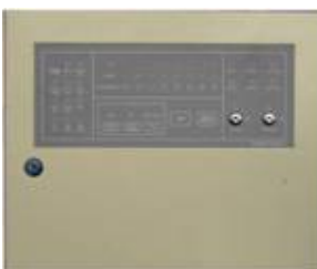
GST108/4 Fire Alarm Panel
