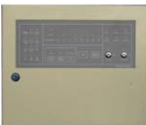
GST108/8 Fire Alarm Panel
