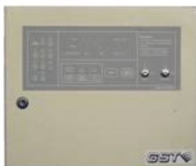
GST102 Fire Alarm Panel
