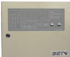
GST104 Fire Alarm Panel
